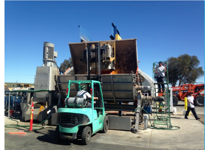
Food Waste Based AD Facility in Sacramento, CA
